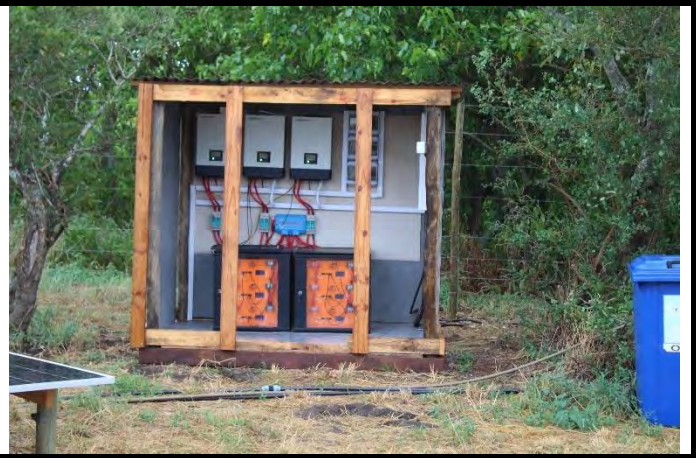
Figure 14: Solar Plant Batteries and Inverters: Awaiting the arrival of a dedicated trailer. Functional.
