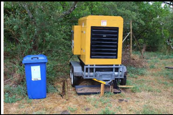
Figure 15: Generator: Back-up for power parked over a drip tray.
