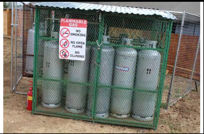
Figure 8: Gas Cage: Locked and stored separately. Good.
