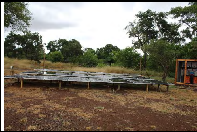
Figure 13: Solar Plant: Functional.
