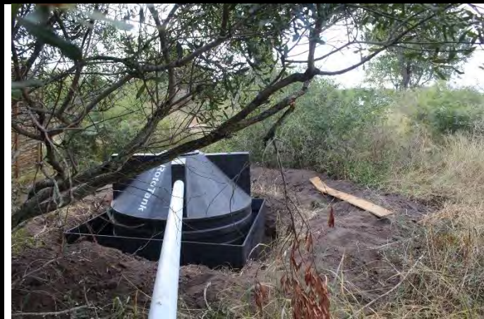
Figure 3: Septic Tanks: Installed to collect sewerage.
