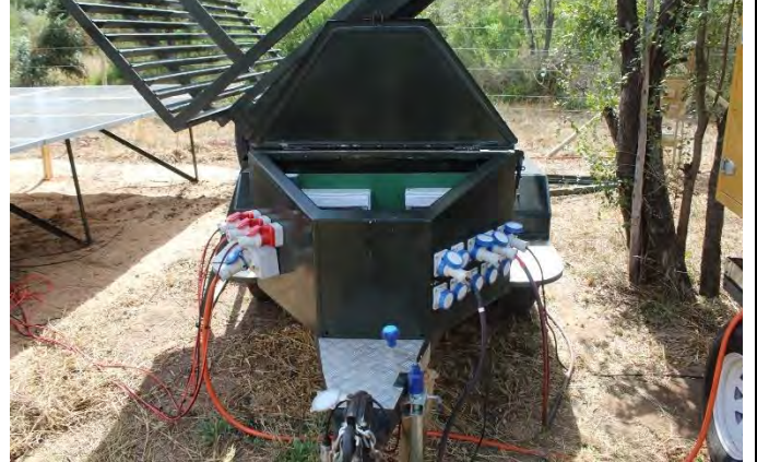
Figure 6: Battery and Inverter Trailer: Mobile and innovative.
