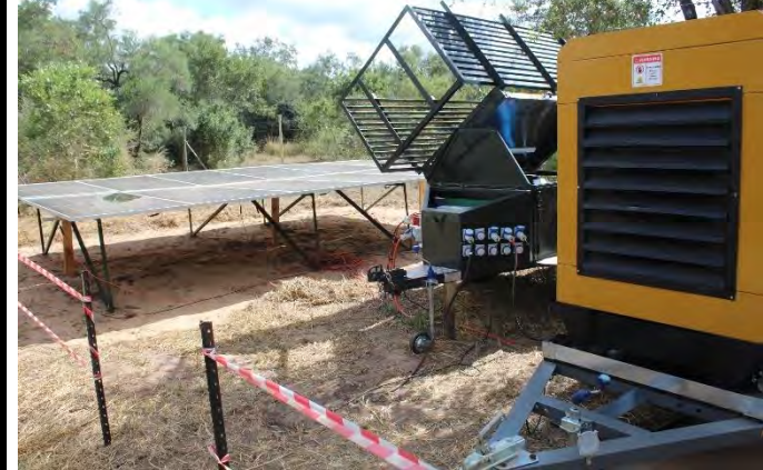
Figure 5: Mobile Solar Plant and Battery Station: Functional.
