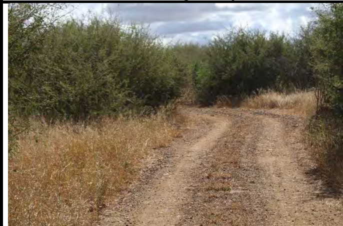
Figure 17: Access Road: Patch gravelling has been used in sections.
