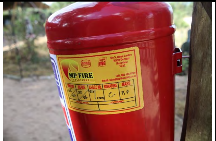
Figure 4: Fire Extinguishers: Erected and serviced.
