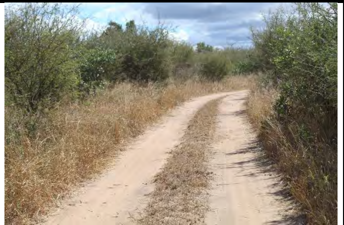
Figure 16: Access Road: Patch gravelling has been used in sections.
