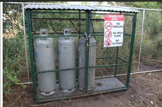
Figure 11: Gas Cage: Locked and stored separately. Clear signage.
