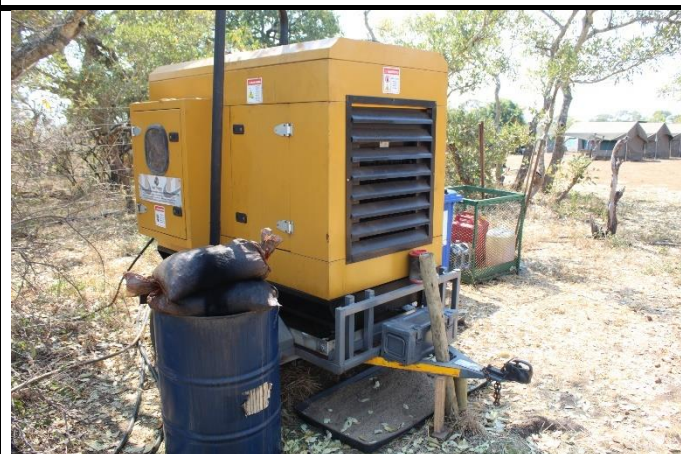
Figure 17: Generator: Back-up for power parked over a drip tray.
