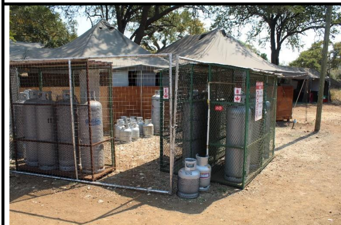
Figure 5: Gas Bottles Facility: Stored separately and locked.
