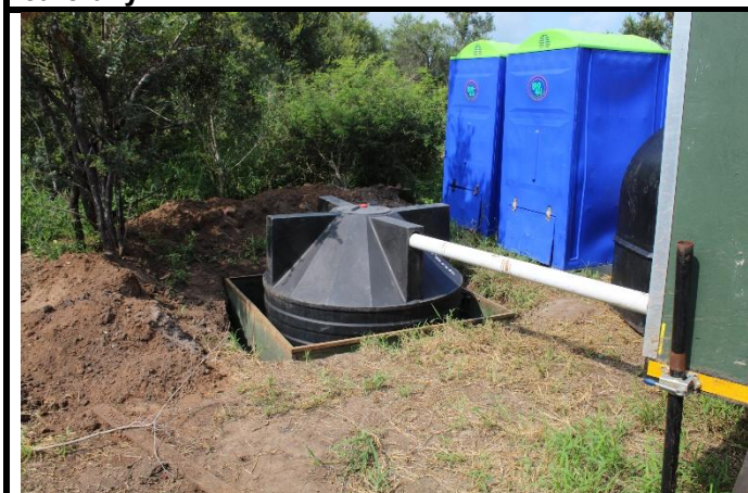
Figure 21: Septic Tank: Emptied every week.
