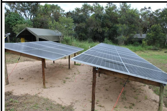
Figure 3: Solar Plant: Producing sufficient power for the camp.
