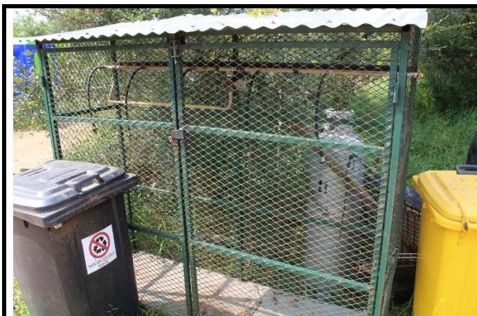
Figure 25: Gas Cage: Safe and secure. Good.
