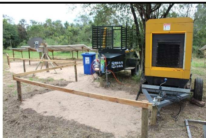
Figure 2: Solar Plant System: Functional. Good.
