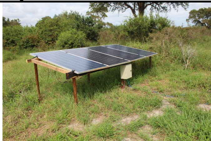
Figure 18: Borehole and Solar Pump: Functional. Pipes will be buried.
