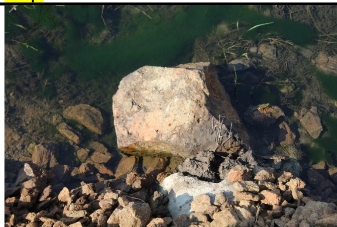
Figure 6: Access Road: Drainage pipes have been installed. Maintain these pipes and remove all blockages regularly.
